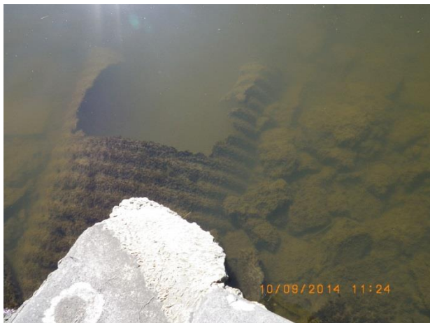
Figure 30 – Corroded metal pipe at outfall 08-284 (minor damage)
