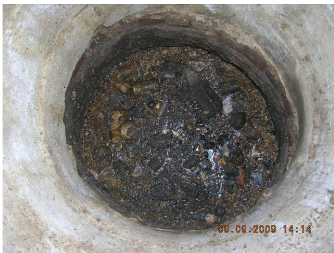
Figure 19 – Floatable debris and grease in upstream manhole 03-81 US1 (2009)
