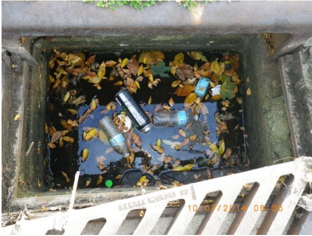
Figure 45 – Minor deposition in inlet 16-142 US1
