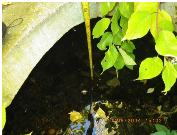
Figure 42 – Minor deposition at outfall 13-3099
