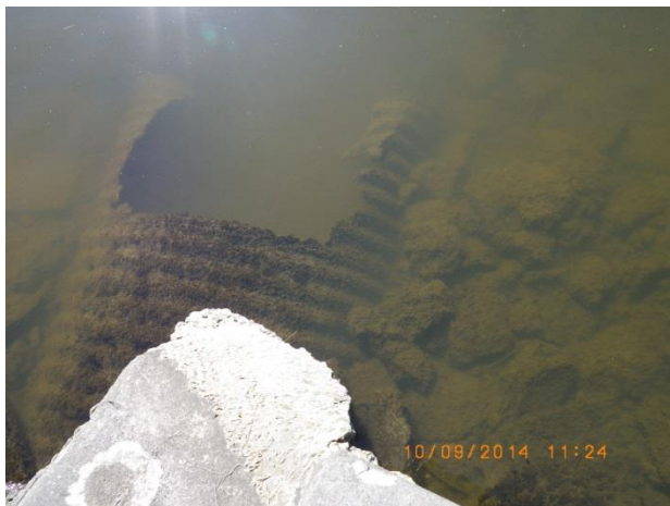
Figure 39 – Minor deposition at outfall 08-284
