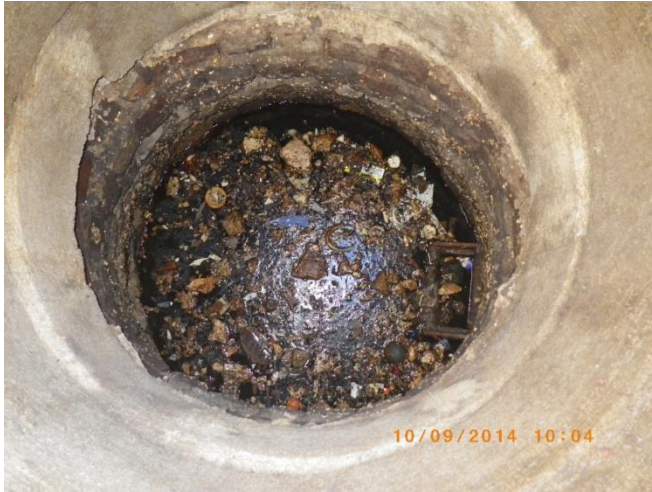
Figure 23 – Oil sheen and debris in manhole 03-81 US1 (2014)
