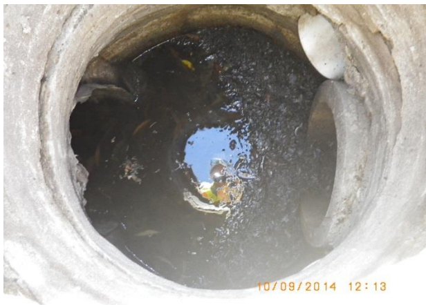
Figure 33 – Minor deposition in manhole 02-322 US1
