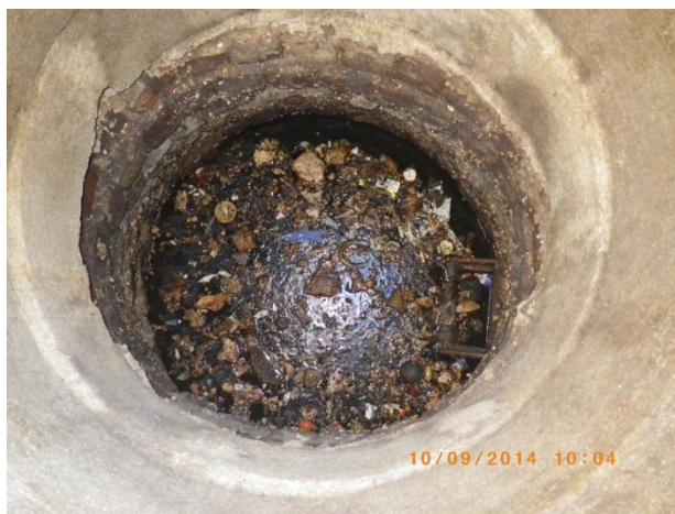
Figure 36 – Minor deposition in manhole 03-81 US1
