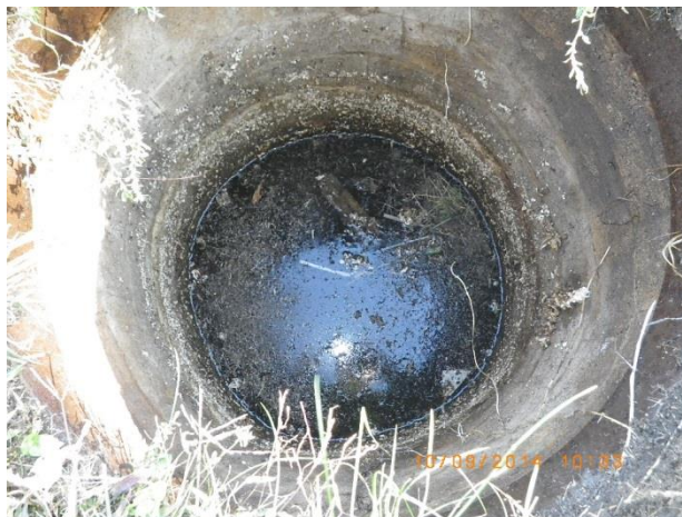
Figure 34 – Minor deposition in manhole 03-35 US1
