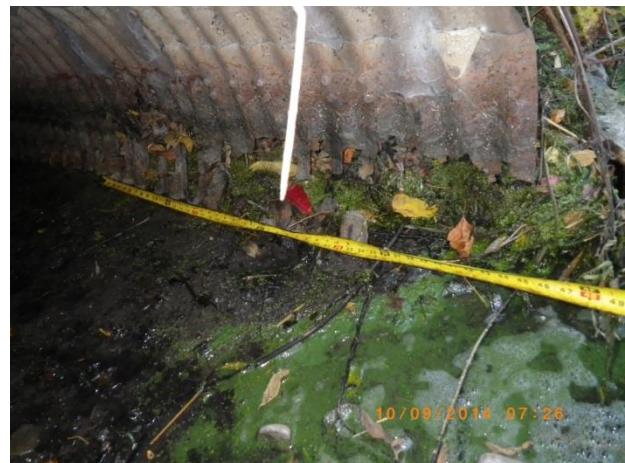
Figure 31 – Corroded metal pipe at outfall 12-890 (moderate damage)
