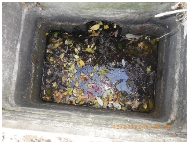
Figure 44 – Minor deposition in inlet 16-119 US1
