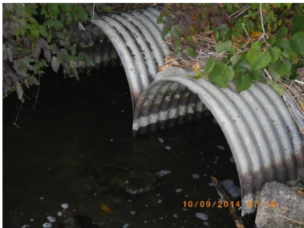
Figure 32 – Corroded metal pipe at outfall 12-890x (minor damage)
