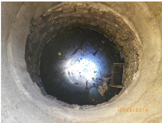
Figure 24 – Oil sheen and debris in manhole 03-81 US1 after vacuuming (2014)
