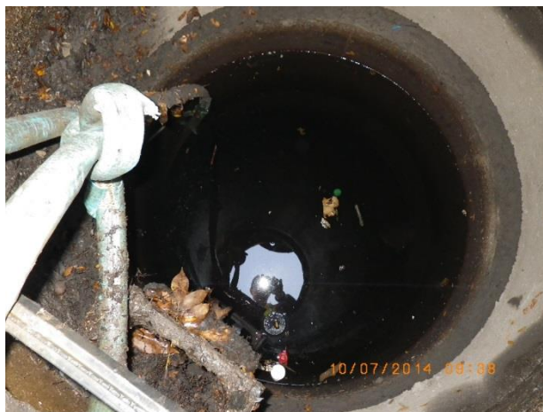
Figure 38 – Minor deposition in manhole 06-221 US1
