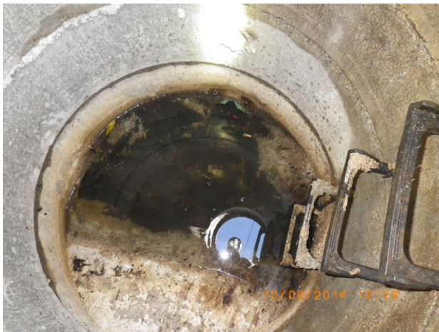
Figure 17 – Pool in upstream manhole 02-184 US1 (2014)
