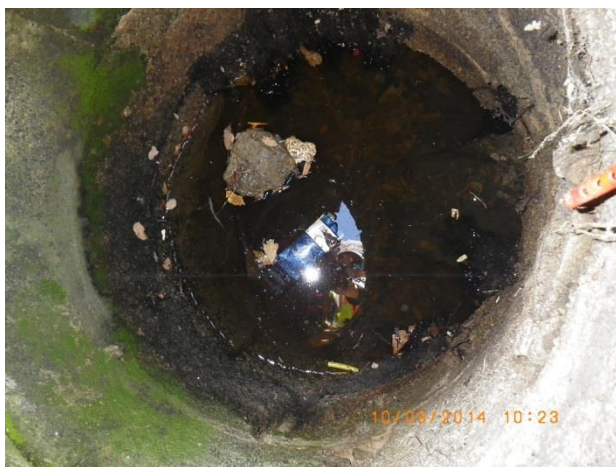
Figure 35 – Minor deposition in manhole 03-381 US1
