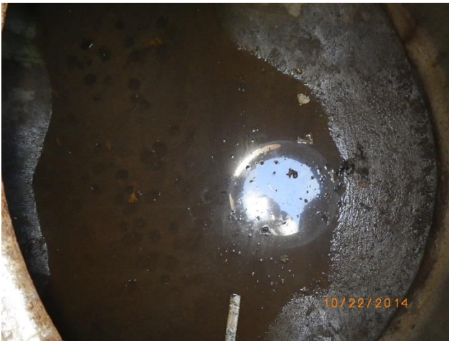
Figure 26 – Petroleum sheen in upstream manhole 03-81 US4 (2014)
