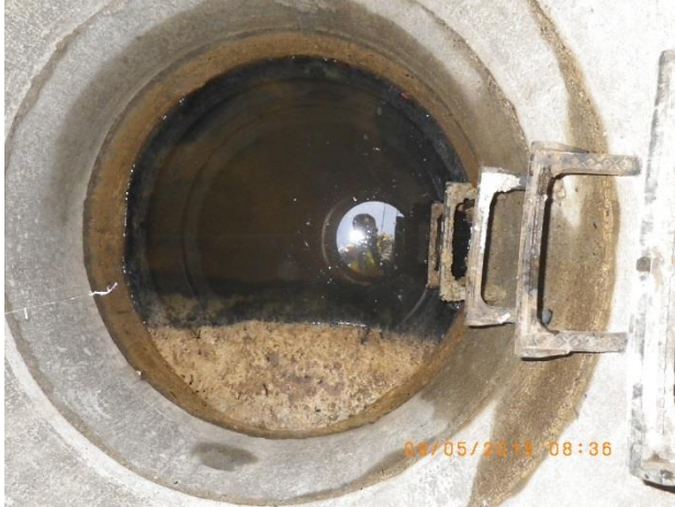
Figure 16 – Pool in upstream manhole 02-184 US1 (2013)
