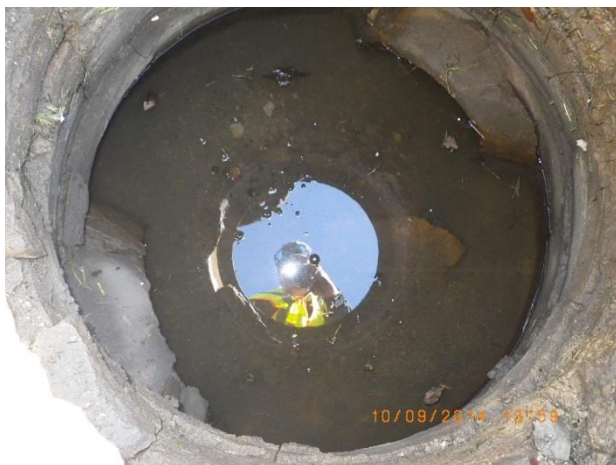
Figure 43 – Moderate deposition in manhole 15-1093 US1
