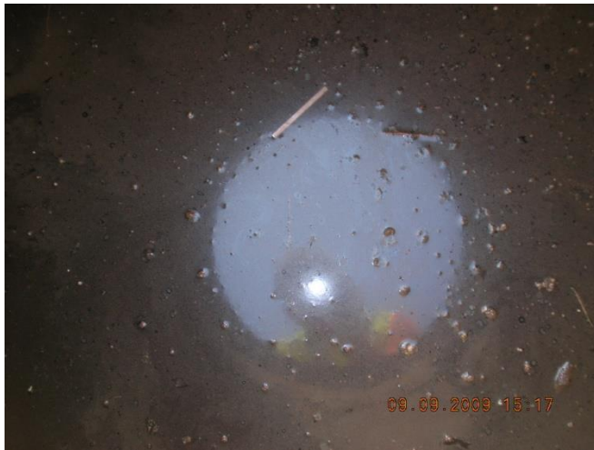
Figure 22 – Oil sheen in upstream manhole 03-81 US4 (2009)
