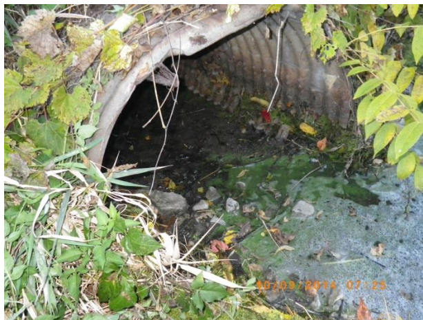
Figure 40 – Minor deposition at outfall 12-890
