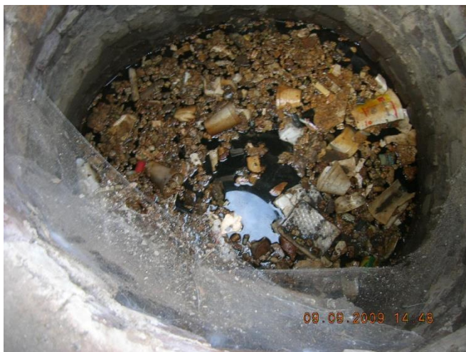
Figure 21 – Floatable debris in upstream manhole 03-81 US2 (2009)
