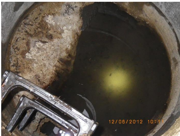
Figure 15 – Pool in upstream manhole 02-184 US1 (2012)
