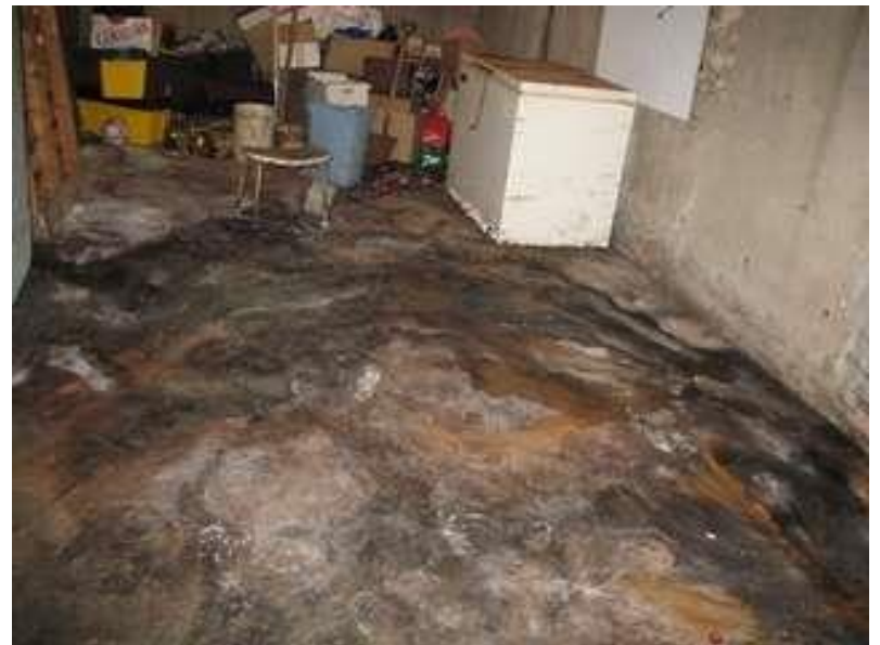
Basement Backups Occurs
