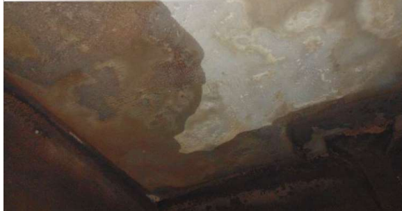
Areas of Damp Shotcrete
