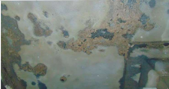
Deteriorated Shotcrete Lining
