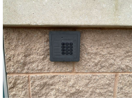
WFP facilities are hardened with locked, solid core doors and electronic intrusion detection.
