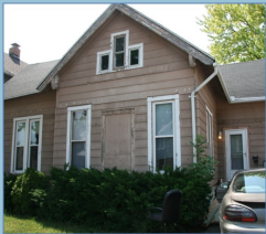
Long term Boarded-up front door
