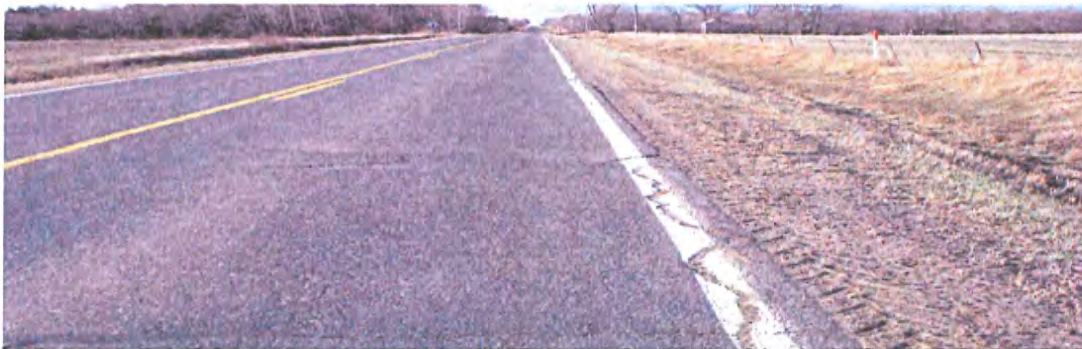
CTH E April – no signs of salt brine residue
