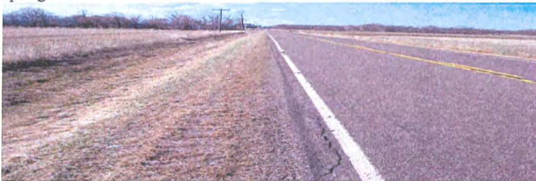
CTH D April – no signs of salt brine residue
