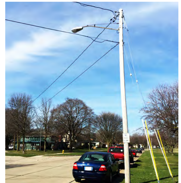
Cobra head light and above ground utilities
