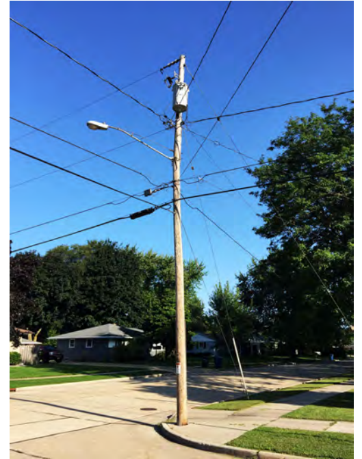
Overhead utility structures
